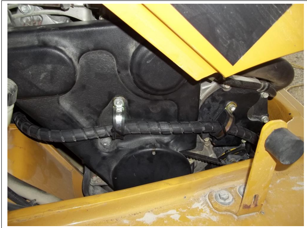
Belt cover re-installed with # 8 AC hose secured and running to the condenser.
